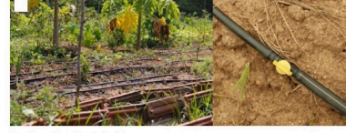
Lateral pipes and taps
